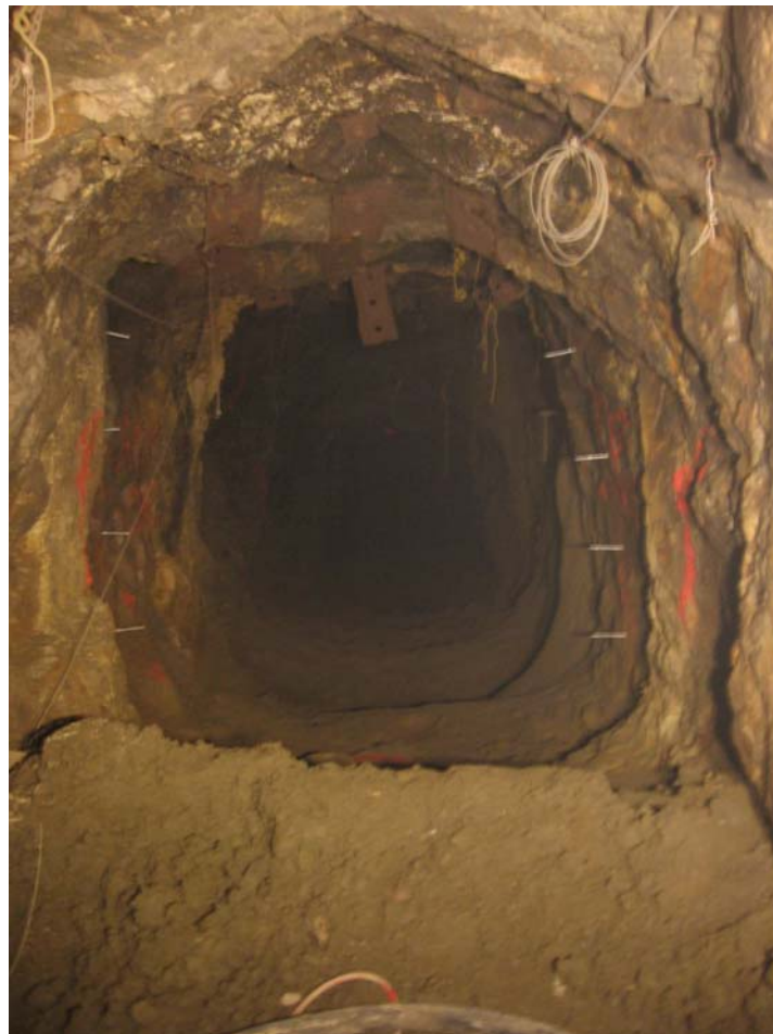
Figure 5. Army Tunnel conditions prior to bulkhead construction (future bulkhead location indicated by sidewall anchor bolts).
