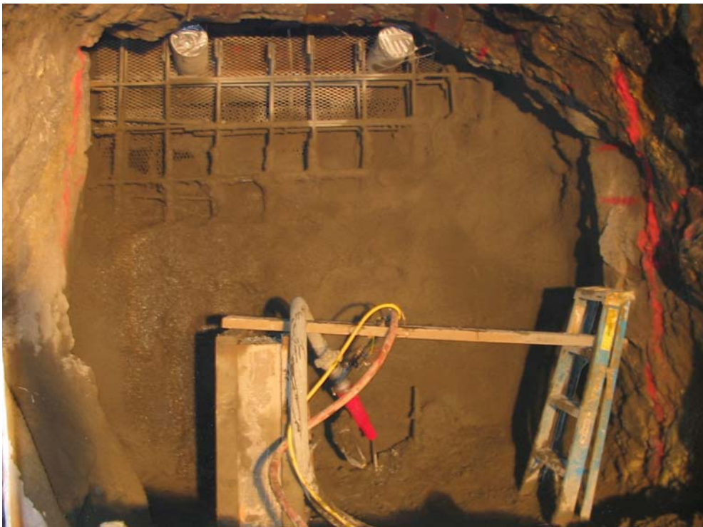
Figure 6a and 6b. Bulkhead conditions during construction (note vent pipes at top of bulkhead).
